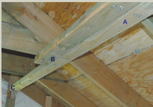
Figure 4-7. In this application of lateral bracing, the 2 x 4s are 18 inches from the ridge and connect to horizontal members that attach to the opposing trusses. Not all roofs will have the horizontal members. The 2 x 4s are connected with two No. 14 3-inch screws (A) and overlap over two trusses (A and B). The end is connected to the gable end with an angle or L bracket (C).
