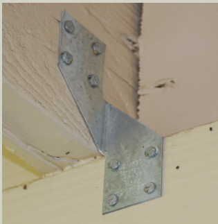
Figure 4-25. This is an example of retrofitting an existing house, originally built without hurricane clips. The popular H3 clip is used here; four nails attach the clip to the roof (truss-rafters) and four more nails attach to the wall or top plate below. For a retrofit, the clips are exposed on the outside of the house; therefore, both the clip and fasteners should be corrosion-resistant and painted to blend with the exterior of the house. With the correct clip and nails, you could perform the work or, if you prefer, hire a licensed contractor.
