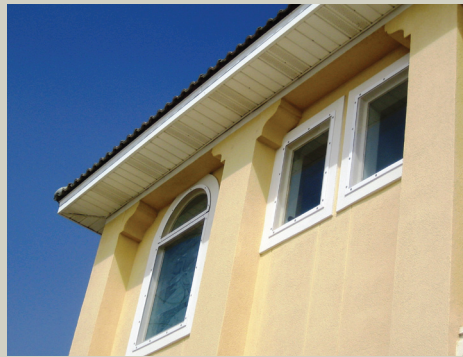
Figure 4-17. Flat impact polycarbonate panels installed directly over windows of a coastal home. This window covering provides excellent storm protection with minimal aesthetic impact. Source: Roll-a-way/QMI.
