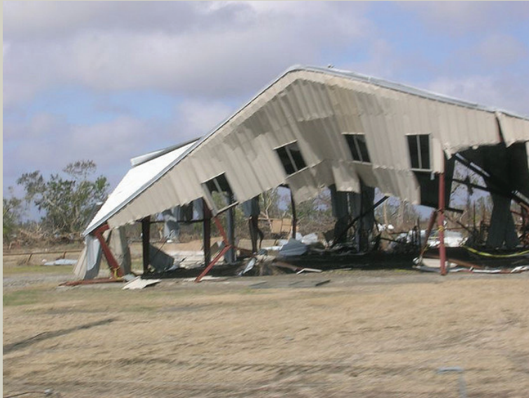
Figure 2-6. Storm surge associated with Hurricane Rita caused damage to properties in Cameron Parish, La. Source: Louisiana Sea Grant.
